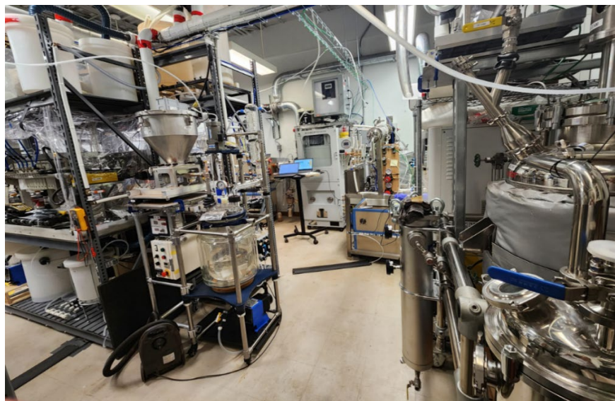
Figure 2: Pilot plant setup at the Boucherville facility
