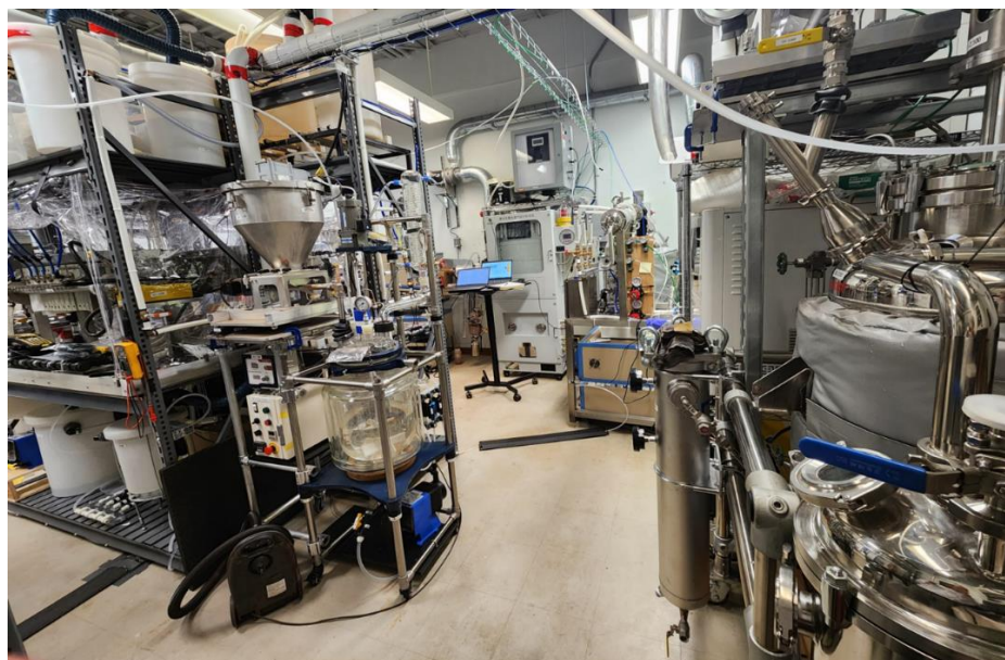
Figure 2: Pilot plant setup at the Boucherville facility
