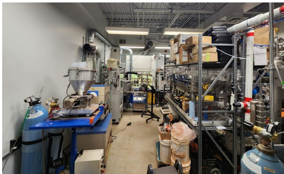
Figure 1: Pilot plant setup at the Boucherville facility
